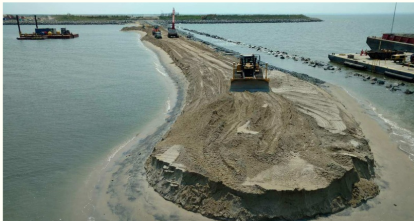
Cell 7 perimeter dike photo credit David Gray (U.S. Army Corps of Engineers)
